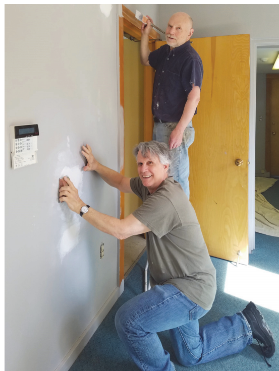
Kenton Rhoades and Chuck Kraemer have been helping to refurbish the Smith Museum entrance area with many tasks, including a new coat of paint.
