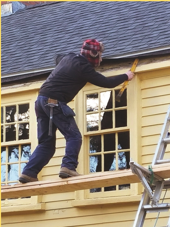
Anthony Arkanson of White Builders prepares the roof prior to installing the new gutter. The new gutters are all wood, as required by our granting agencies. The wood is fir, and the gutter will be later lined with copper.
