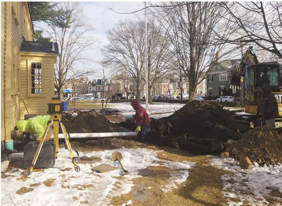
Workers from Koster and Sons Excavating lay piping in the Jason Russell House yard. This piping will direct water from the new gutters and downspouts to a newly-constructed drywell beneath the lawn.
