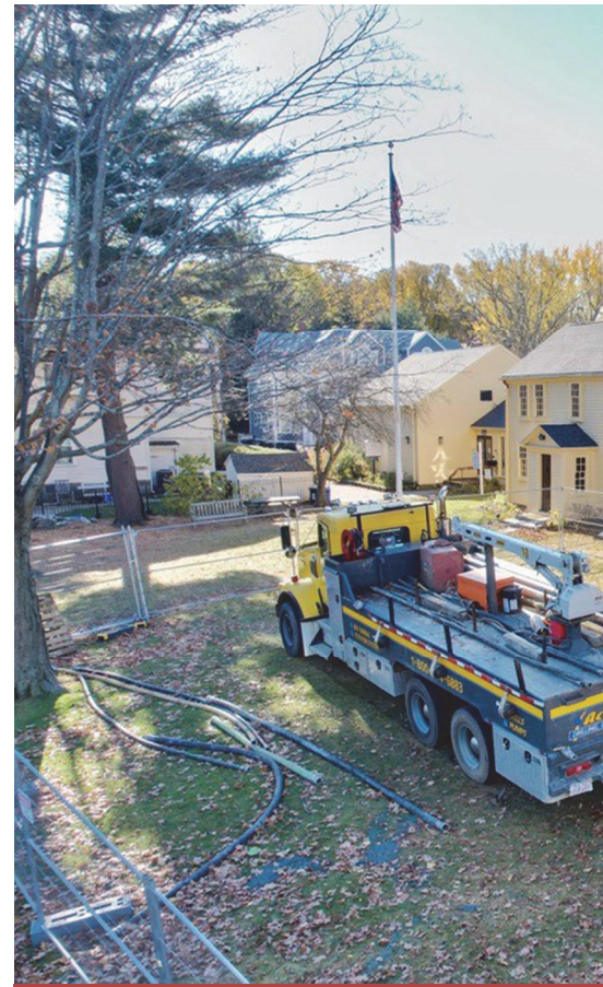
Well drilling rigs on the lawn of the JRH. Photo courtesy of
